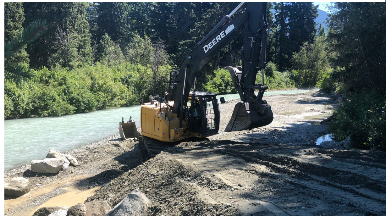
Photo 3: Gravel Bar #19 preparing for excavation. Building a ramp for truck ease of access during excavation.
