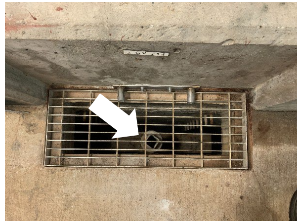
Photo #2: Effluent Gate Valves below grade at back end – use water key to open/close
