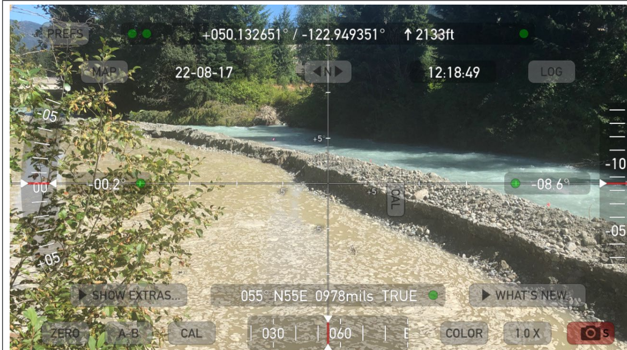
Photo 1: Gravel Bar #15 excavation complete – facing downstream. Berms still intact with no creek flow through excavation area.
