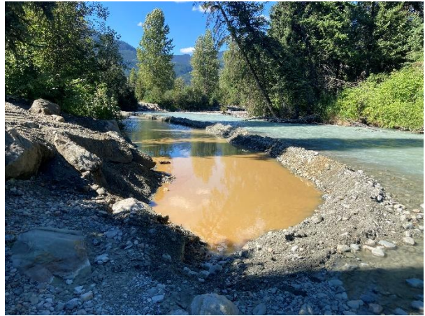
Photo 8: Looking north at the access ramp and constructed berm of Bar 17. August 22, 2022.
