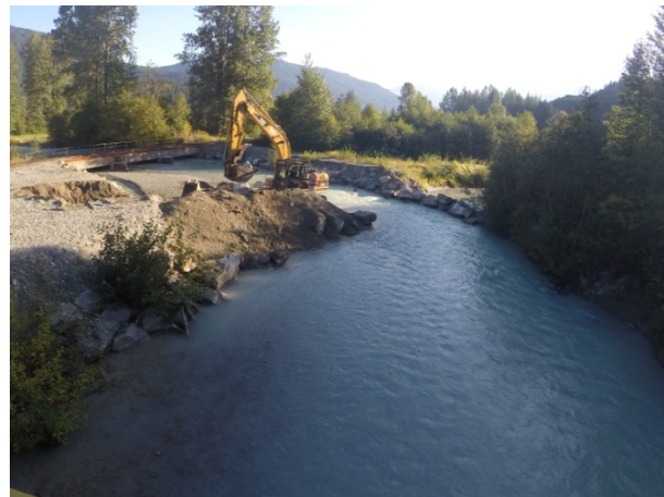
Photo 6: Constructing berm bridge from river left across to river right diversion channel
