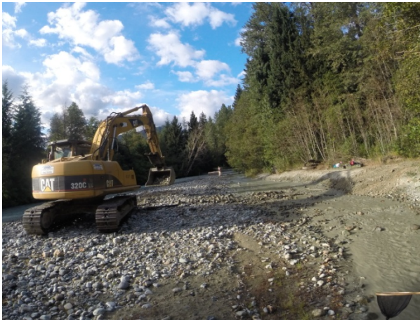
Photo 3: Excavator crossed side channel to gravel bar preparing to construct isolation berm
